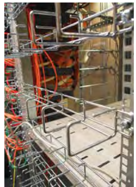
Flexible cable management options, racks and cabling have full access from all sides.
